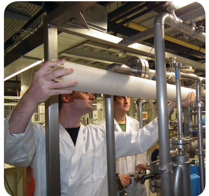
Three-stage pilot system (RO/NF/NF) with five 4" membrane modules
